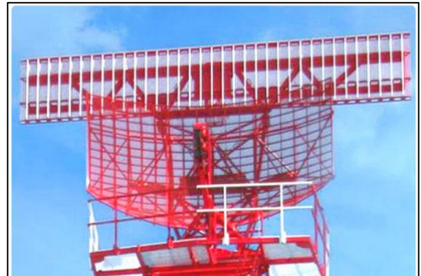
Figure 1. SkySearch-3000 co-mounted PSR, SSR.
